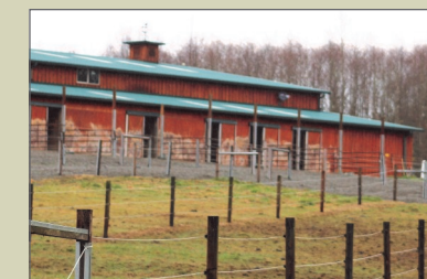
Gravel and a concrete pad outside of the horse stalls control mud and runoff.
